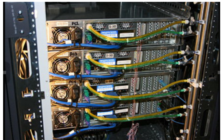
Figure 3. Rear View of a Server Rack with a Chillydyne Cool-Flo Liquid Cooling System [6]
