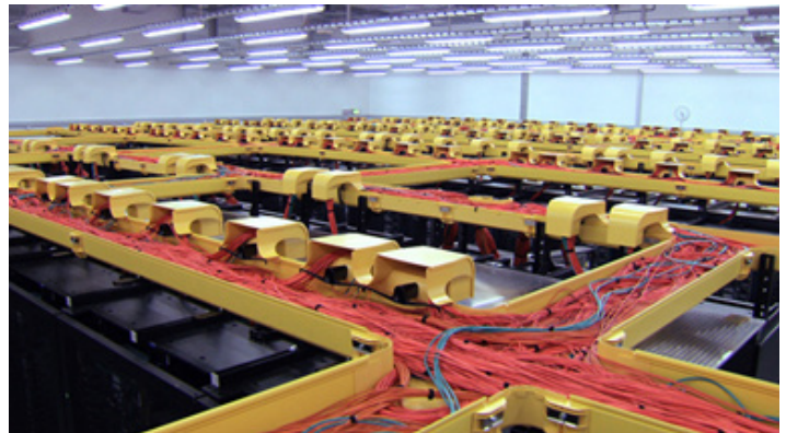
Figure 3. SuperMUC Cooling System Allows a Higher Inlet Water Temperature and Resulting Hot Outlet Water is Used to Heat Buildings [6]
